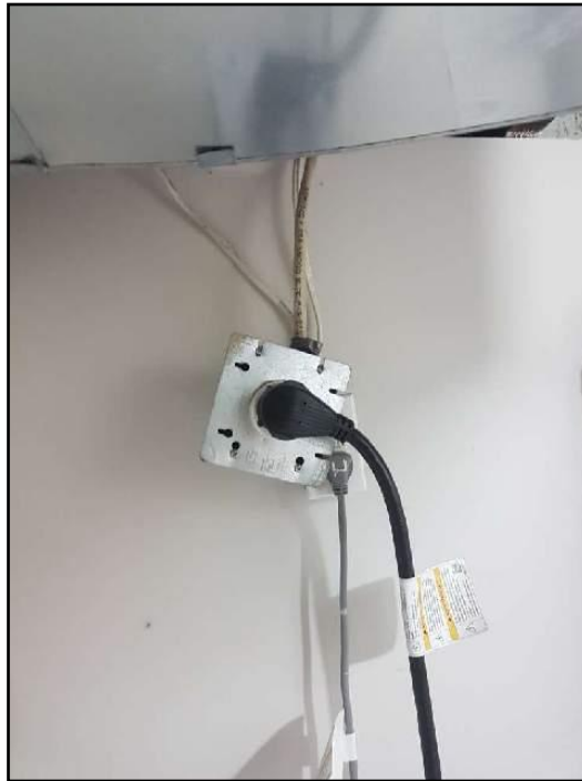
7. Not well secured
