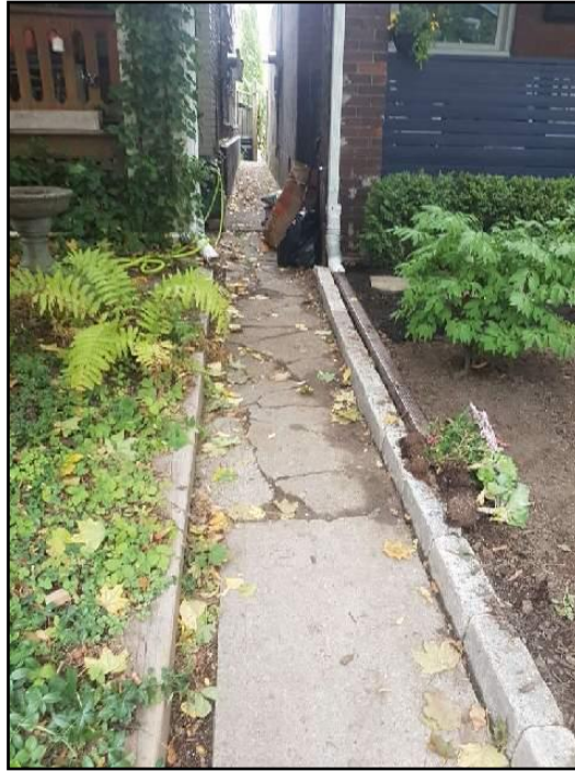
5. Cracked or damaged surfaces
