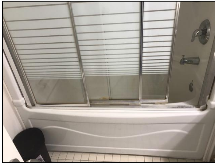
Faucet, diverter and doors - loose
