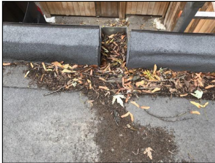
Roof drain/scupper - vulnerable area...
