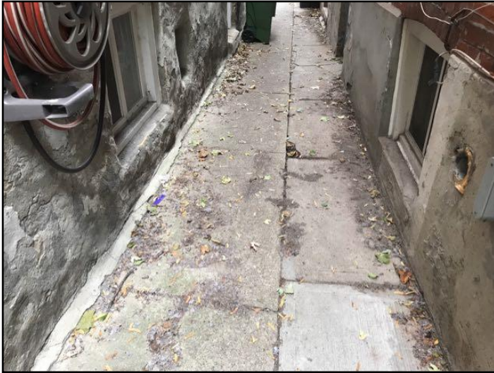
Improper slope or drainage
