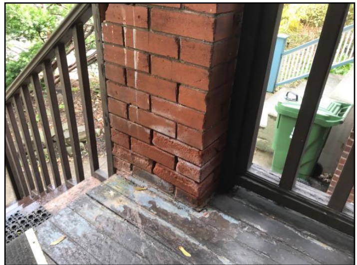
Masonry and mortar - deteriorated/missing
