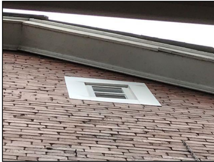
Arches or lintels - not visible/missing
