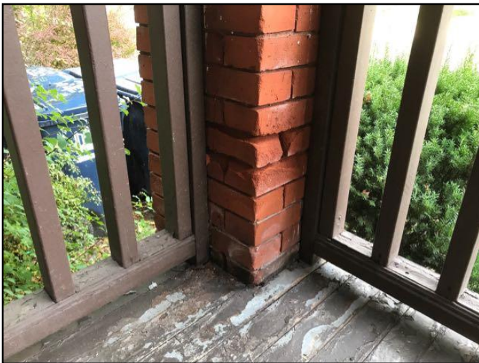
Masonry and mortar - deteriorated/missing
