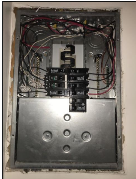
Breakers - Third floor hall
