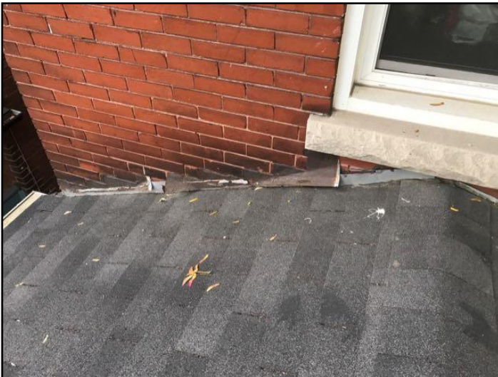
Flashing - damage/missing, leak
