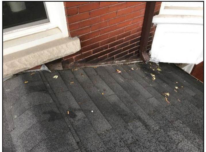
Flashing - damage/missing, leak
