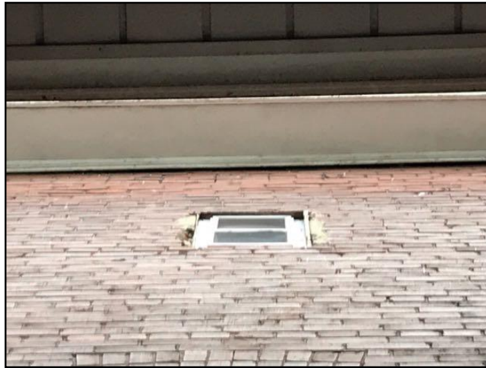
Window - installation incomplete...
