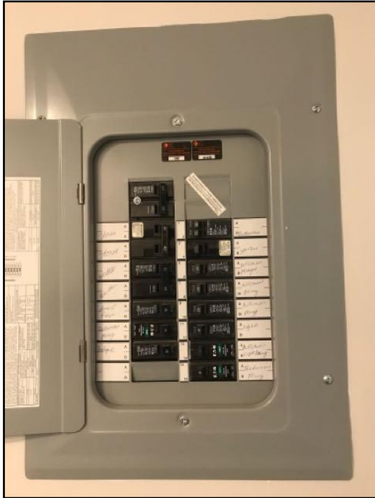
Breakers - Second floor hall
