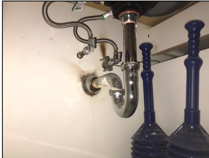
Trap - rust, leak
