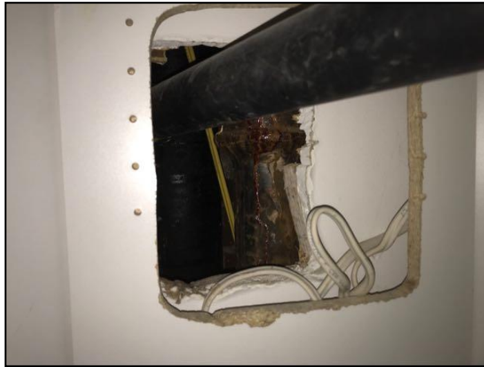
Waste piping - rust, leak suspected
