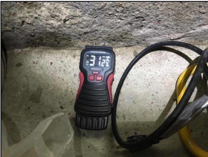
Dampness, efflorescence, water stains
