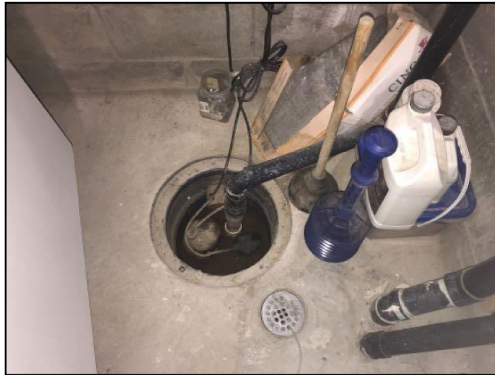
Sump pit and pump
