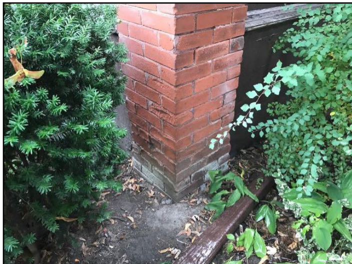
Masonry and mortar - deteriorated/missing
