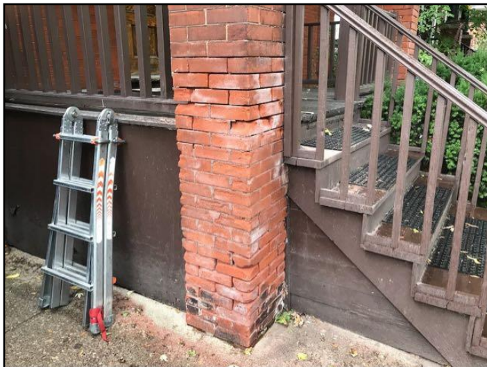
Masonry and mortar - deteriorated/missing
