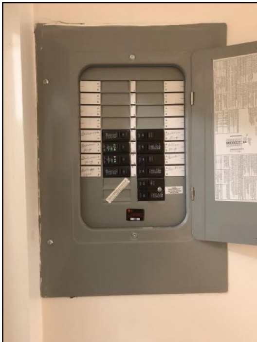
Breakers - Third floor hall
