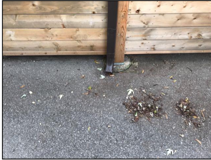
Discharge location poor
