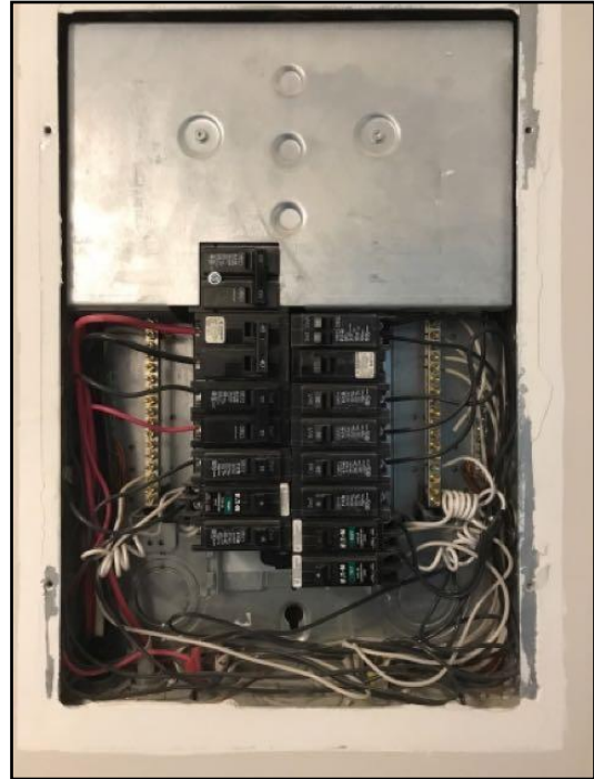
Breakers - Second floor hall
