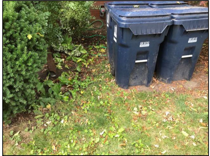
Improper slope or drainage
