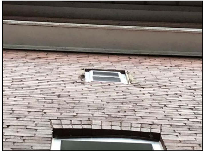
Arches or lintels - not visible/missing
