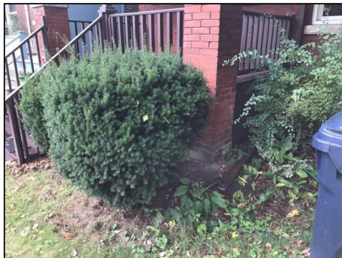
Porch - access restricted underneath
