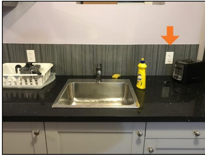
GFCI outlet (20 amp) - redundant
