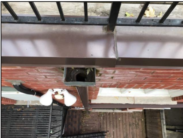
Roof drain/scupper - vulnerable area...
