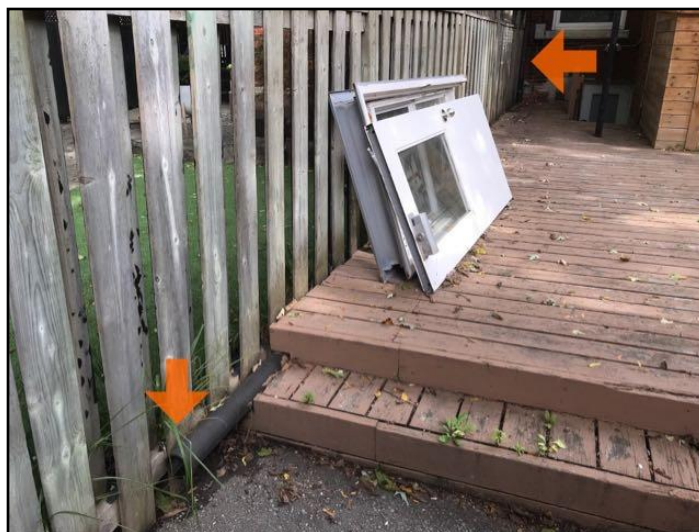
Extension - length excessive, slope suspect
