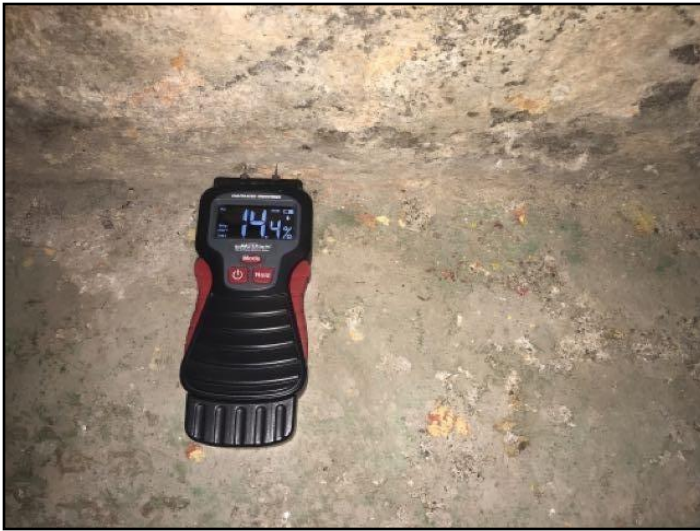
Dampness, efflorescence, water stains
