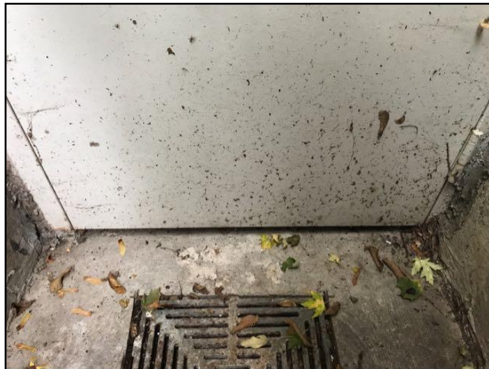
Threshold - clearance inadequate
