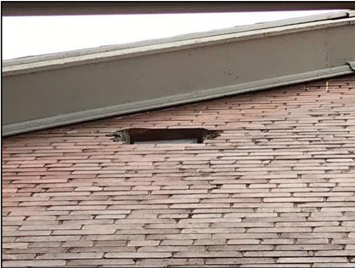
Arches or lintels - not visible/missing
