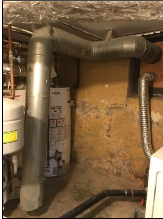
Combustion air supply-installation incomplete
