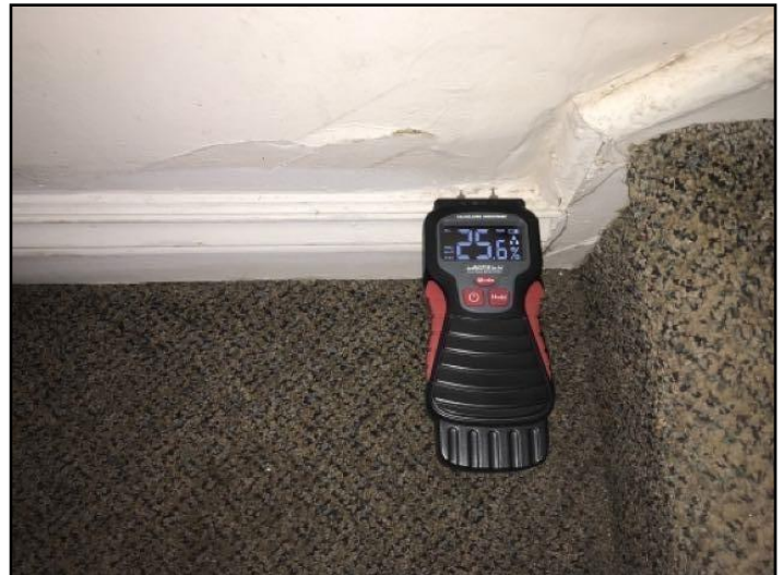
Dampness, water stains/damage
