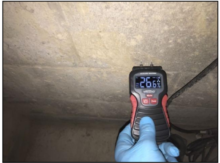
Dampness, efflorescence, water stains
