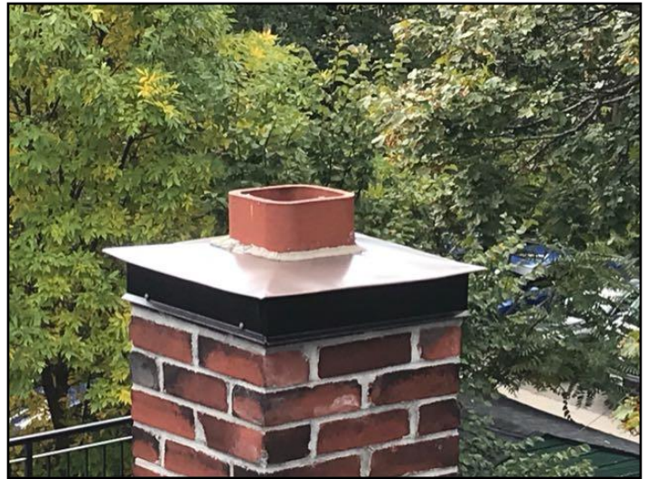
Weather cap - missing
