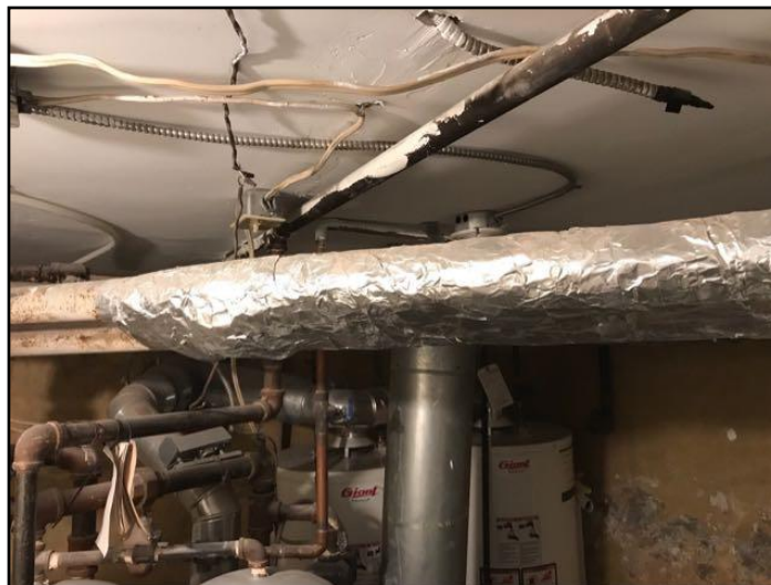
Piping insulation - may contain asbestos
