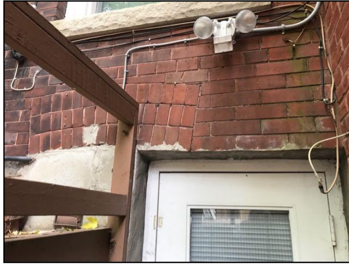
Lintel - not visible/missing
