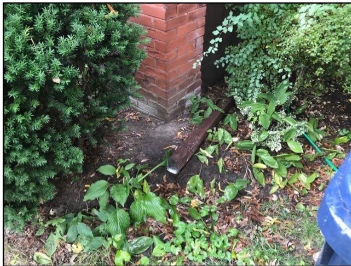
Discharges too close to masonry column
