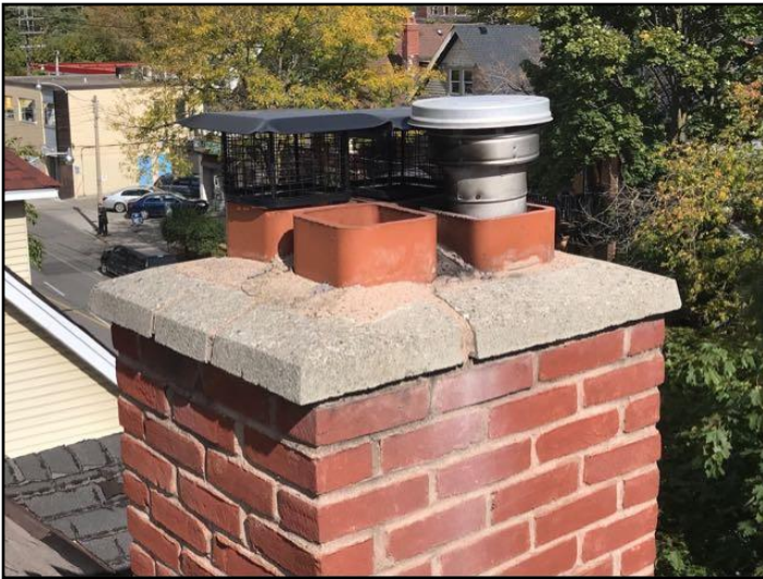
Weather cap - missing
