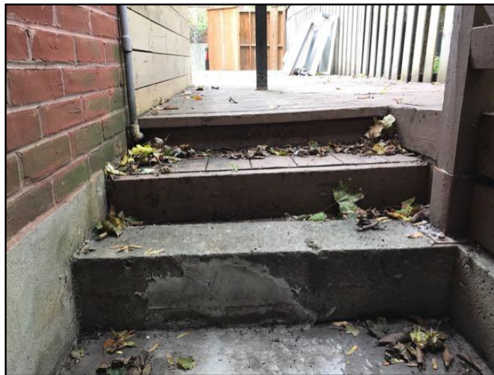
Stairs - riser height uneven
